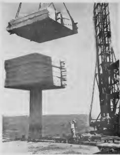
At Lake Maracaibo, where most of Lago's oil comes from, enormous weights are used for pulling cement piles into the lake bottom. The derricks are erected on these piles. (Photograph by Vachon)
